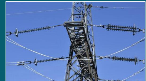
Vattenfall | 2024-2026: Power lines in Södermanland to supply electricity to SSAB's steel mill in Oxelösund
