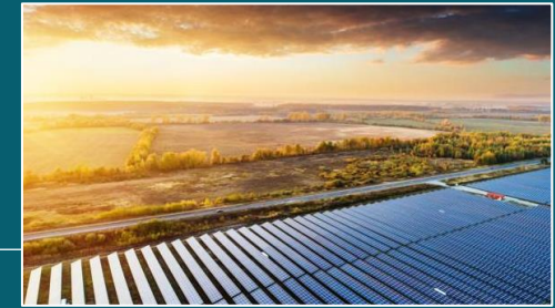
Skarta Energy | 2023-2026: Constructing a large-scale 102.5 MWp solar farm in Utajärvi, northern Finland
