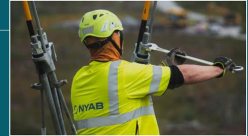
Svenska kraftnät | 2022-2026: 90 km of the 400 kV transmission line between Sweden and Finland
